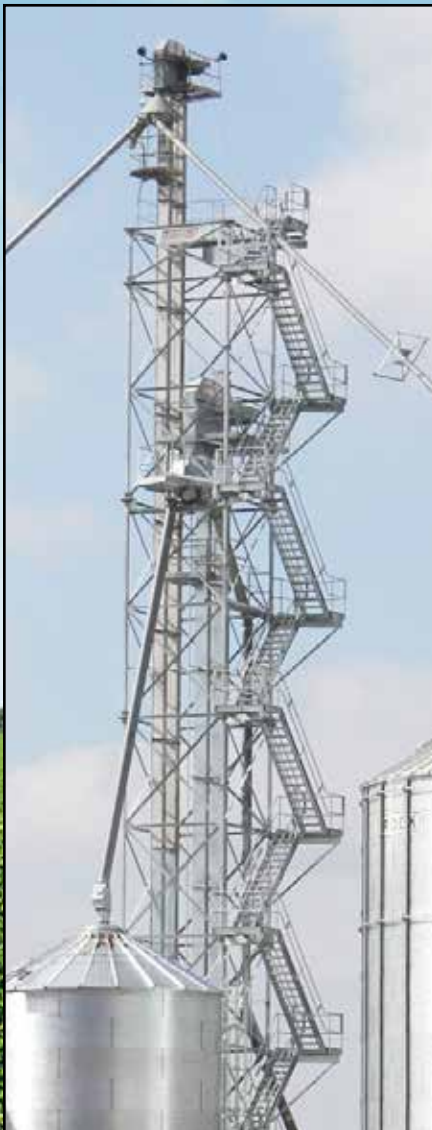
Service Stairway and Custom Walkways to Varying Height Elevator Platforms
