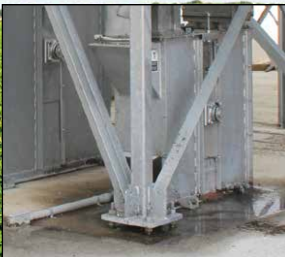
Tower Anchor Plates
