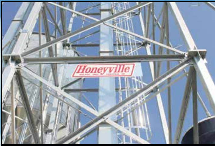
125' Tower: Dry Elevator Inside, Wet Elevator Outside and Service Ladder on Elevator
